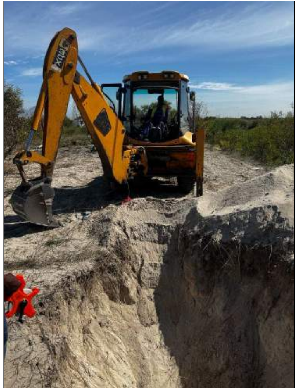
Soil Spoils as observed outside TP1
