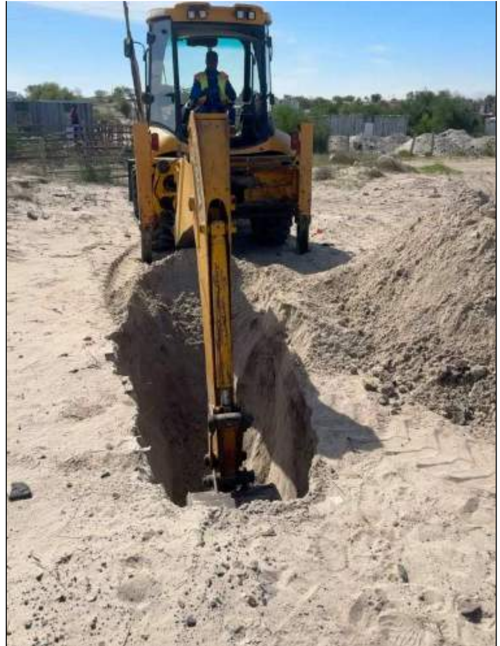
Soil Spoils as observed outside TP2
